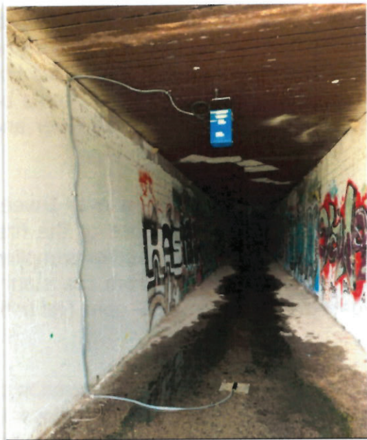
Figure 6a. Flow Meter Installation Site
