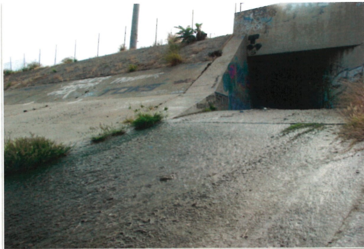
Figure 3: Eagle Rock Storm Drain Outfall at LA River with Dry Weather Flow, Adjacent to G2 Site.
